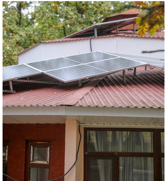
Solar panels installed by Ormax at RAC
