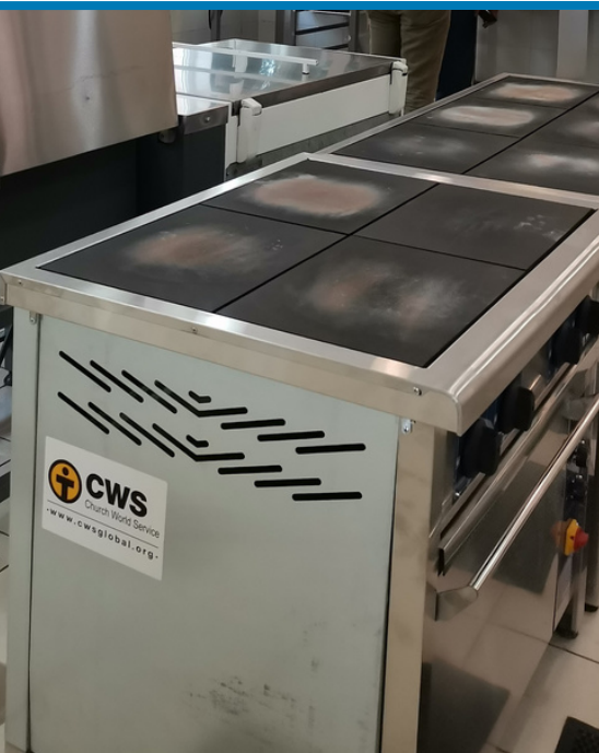
Kitchen equipment in a RAC
