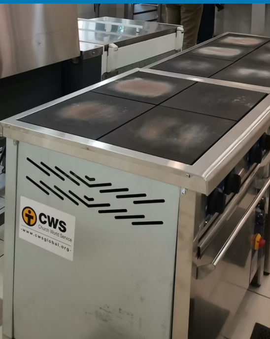
Kitchen equipment in a RAC
